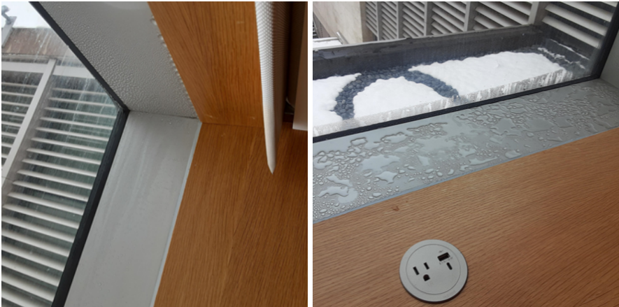
Two photos showing Winter 2024 conditions. Head on left. Sill on right.
